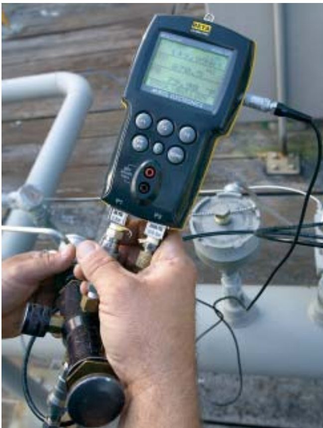
Gas Flow Calibration/Custody Transfer
